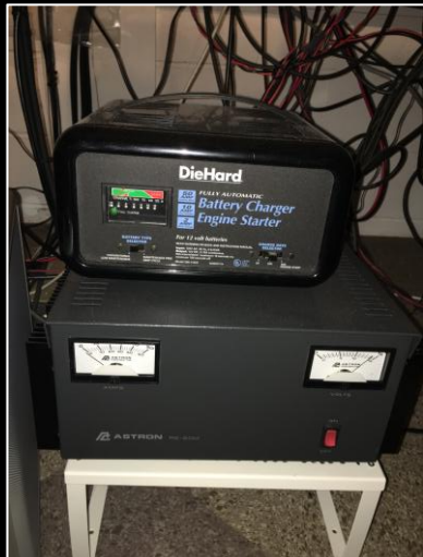
Station Power & Boost Charger
